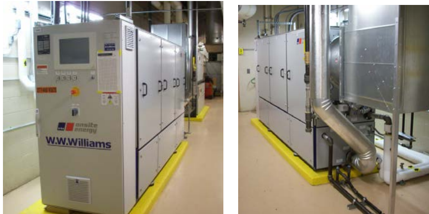
Figure 6a. CHP Unit (front and back views with heat recovery piping)
